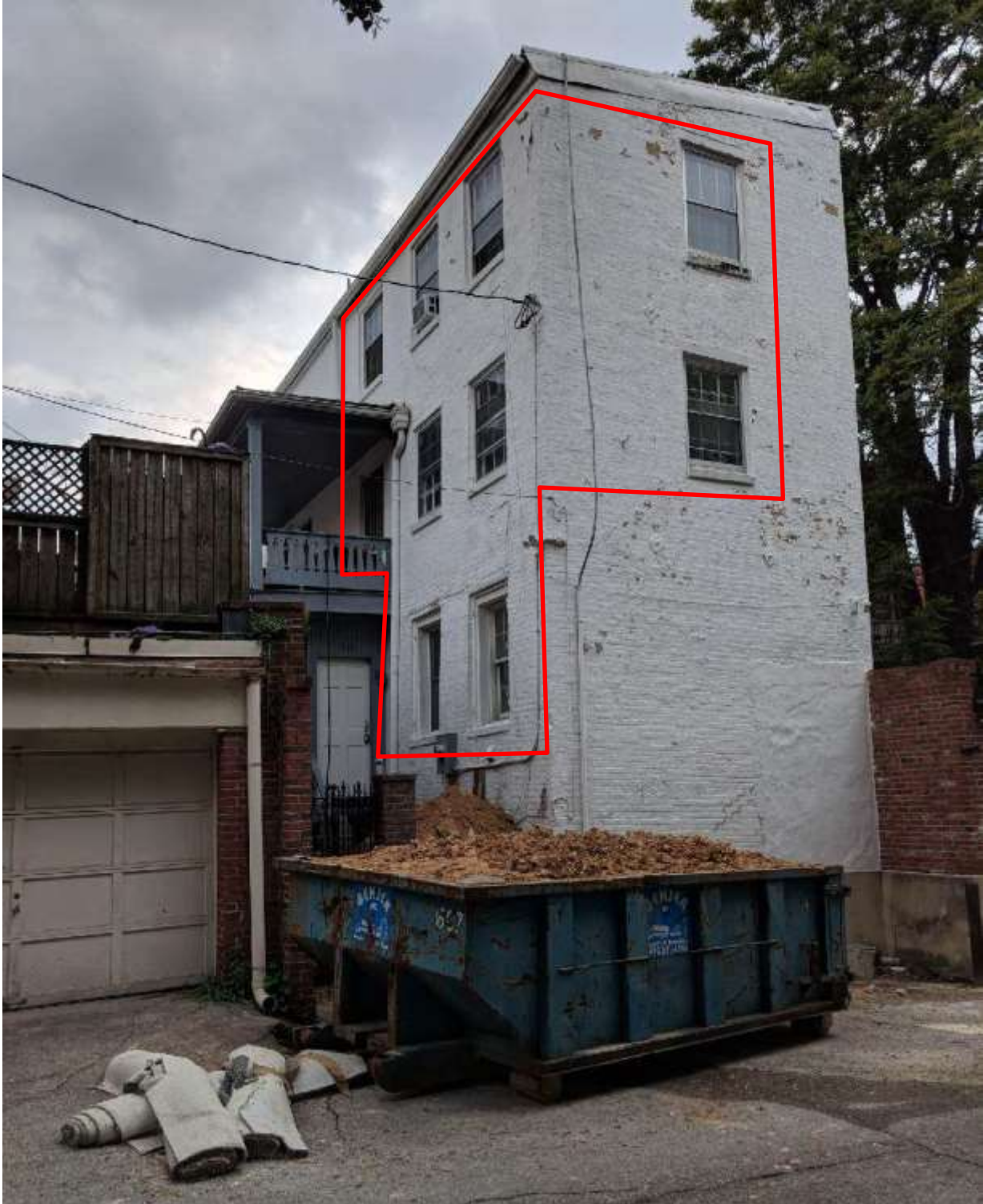
Image 8: Rear elevation from Jordan Street, highlighting the ten windows that are highly visible from this public right-of-way. All of these windows have been replaced sometime in the past 30 years without CHAP approval or building permits.
