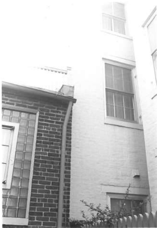
Image 6: Photograph of rear windows from 1980, demonstrating a mix of wood windows from several eras, including a 2/2 and 1/1 window, indicative of the late 19 th and early 20 th centuries. The 6/6 windows are likely early 20 th century replacements. On the far right windows, note the lambs tongue lugs on the meeting rail, indicative of a late 19 th /early 20 th century window.
