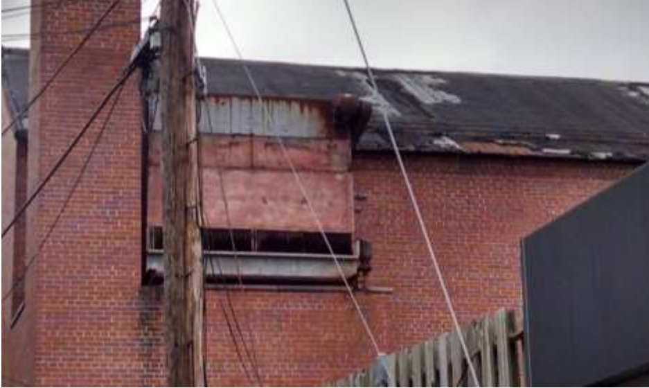
Side, showing deterioration of roof, June 2016.
