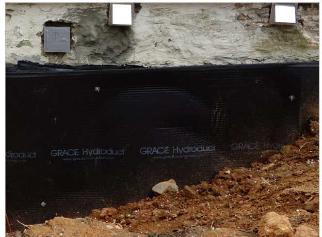
The structural integrity of masonry walls should be verified prior proceeding with dry floodproofing. All sealers should be concealed by soil or historically appropriate material based upon location.
