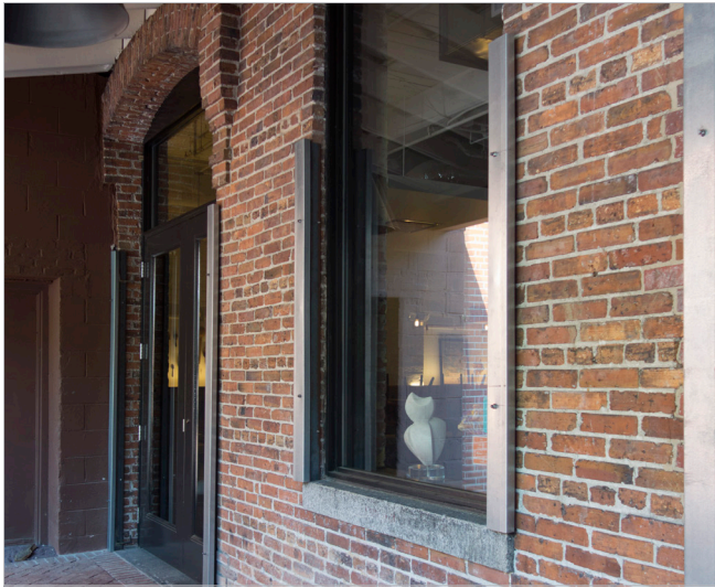
The metal frames flanking the window and door openings are used to hold flood barriers in place.
