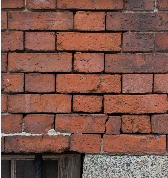
Although brick has an acceptable flood resistance, deteriorated brick and the lack of mortar can significantly reduce the resistance level.
