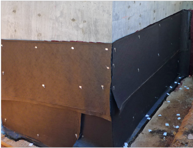
Concrete buildings are generally good candidates for dry floodproofing because of their ability to withstand loads and their smooth surface for the application of sealers.
