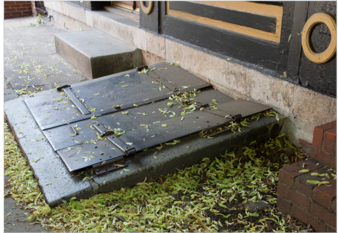
The flood vulnerability of all potential building entrances should be evaluated and addressed to minimize potential damage.
