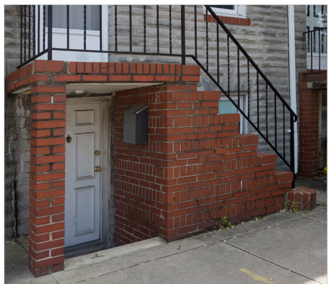
The entrance door is located below the sidewalk height. As a result, the lower level might be more vulnerable to flooding than what the FIRM may suggest.
