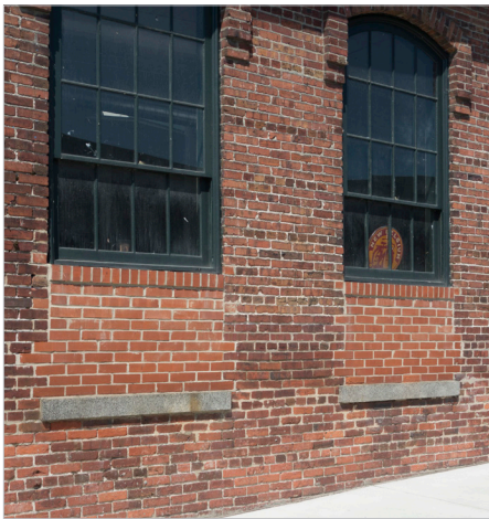
After persistent flooding, the lower sections of the windows were infilled to improve flood resilience. The infilled windows retain their historic sills, and replacement sash are sympathetic to the original configuration.
