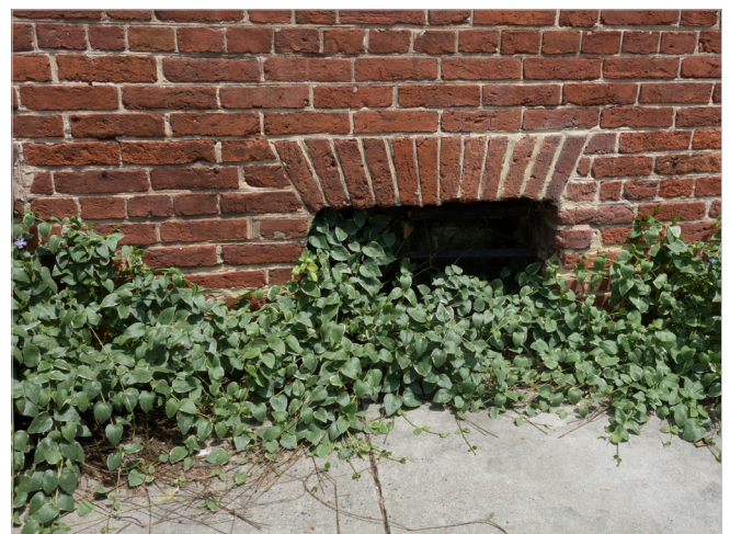
Maintenance includes the removal of vegetation that can damage building materials, obscure openings, or trap debris.
