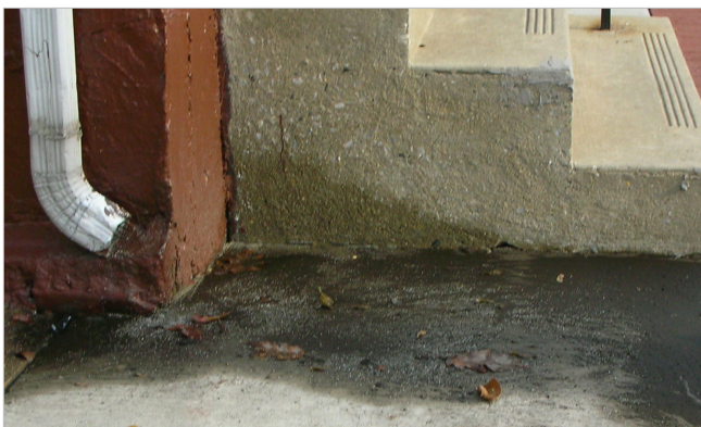
Downspouts should be kept clear and the surrounding ground sloped away from the building foundation to minimize potential water damage.
