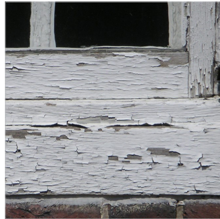
Open joints around windows and door frames can provide a path for water infiltration. Regular replacement of sealant is required for it to retain its effectiveness to prevent water infiltration.
