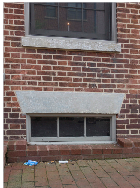
Screening obscures the interior storage at the first floor at the wet floodproofed rowhouse pictured above. The former basement has been infilled with gravel that has been visually obscured through the lower window opening.
